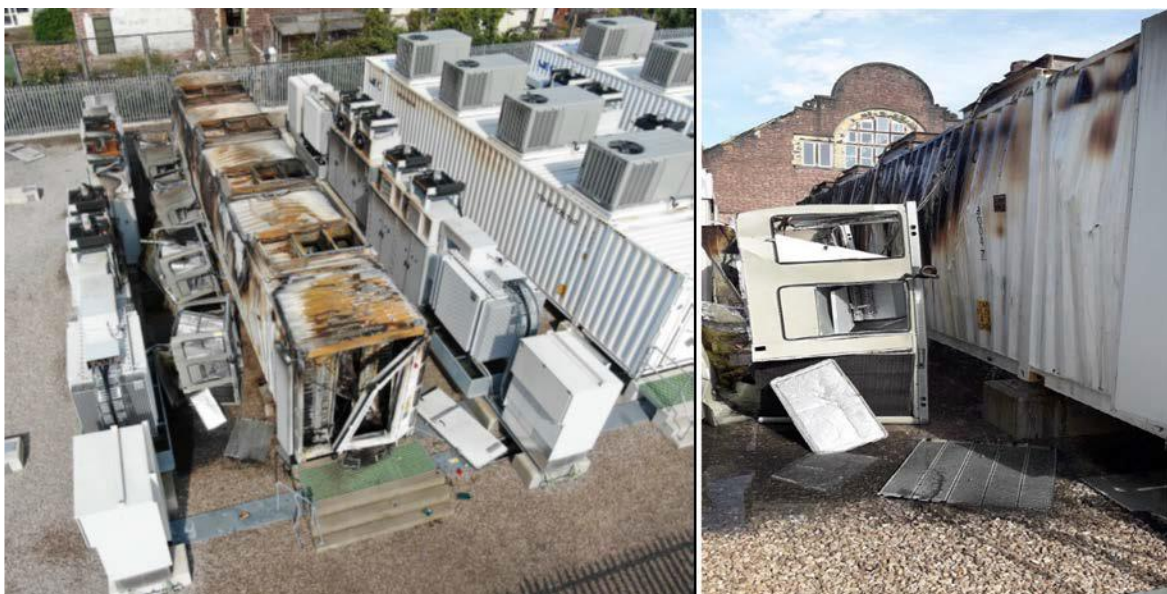
Figure 6 – Post incident photographs 11
