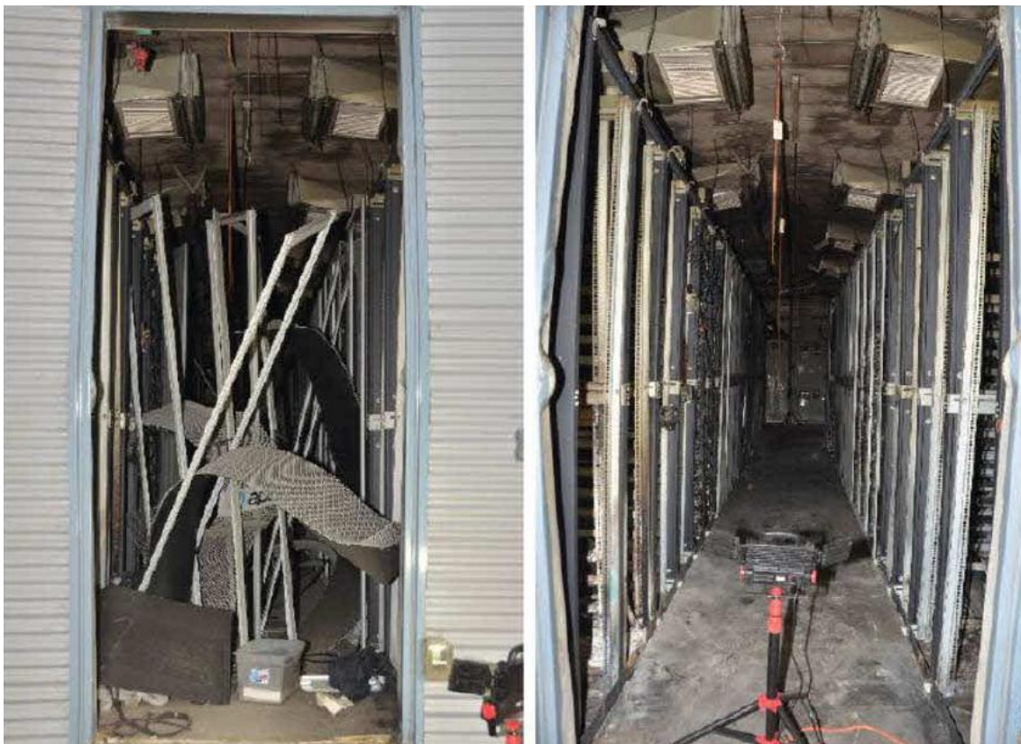
Figure 4 – BESS contained post deflagration event 7
