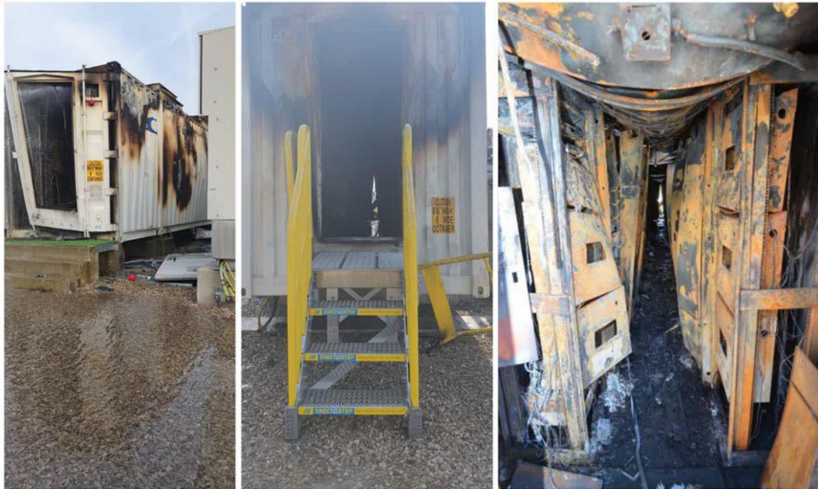
Figure 7 – Post incident photographs 12
